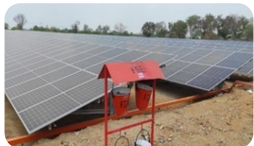
1.53 MW at Krishnapuram unit
