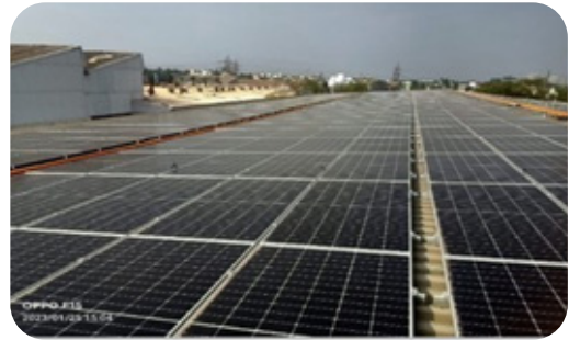
0.41 MW at Padi unit
